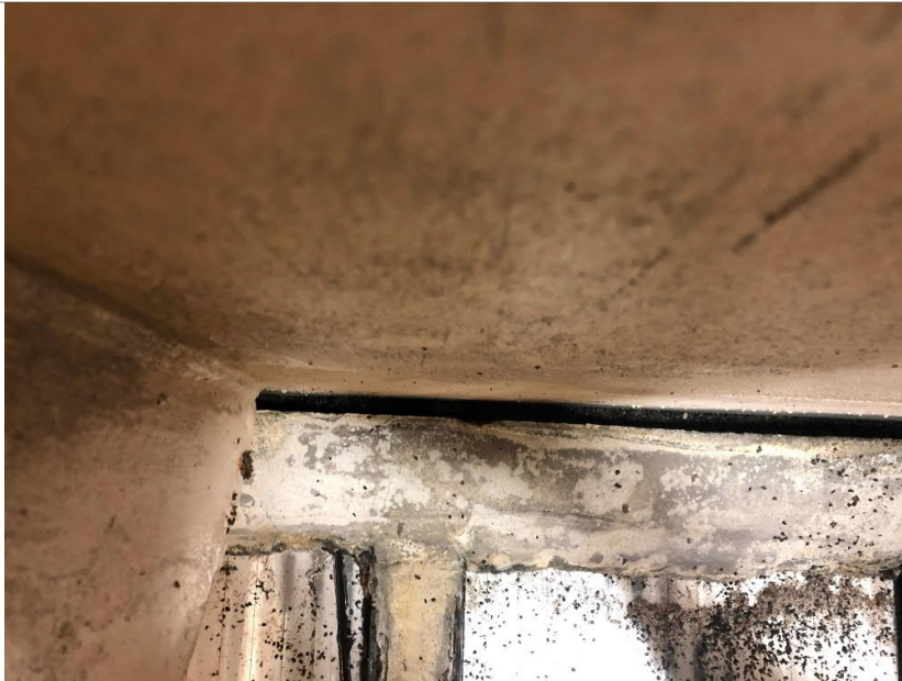
Gap between end of underdrain laterals and tank wall near AC section of Trident
