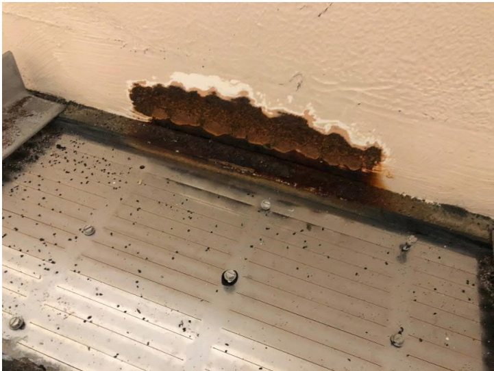
Example of the need for re-coating of tank interior. Near center flume of filter.
