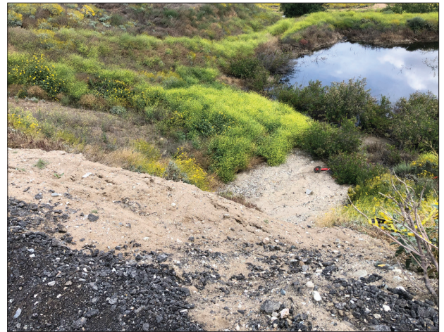
(Above) Looking north at Alder at failed road area (Below) Looking east downhill on Alder at failed road area
