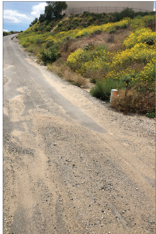
Looking south at Reservoir 3-1 access road with sediment
