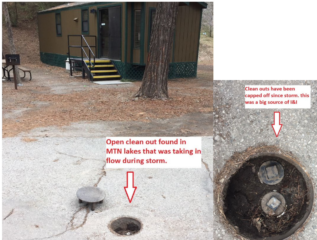
Figure 4-1. Clean out at Mountain Lakes Where Storm Water Infiltrated in February 2019
